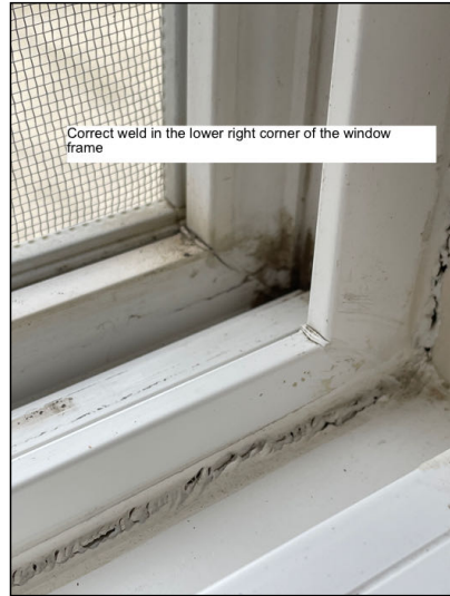
Cracked. Not Correct.
