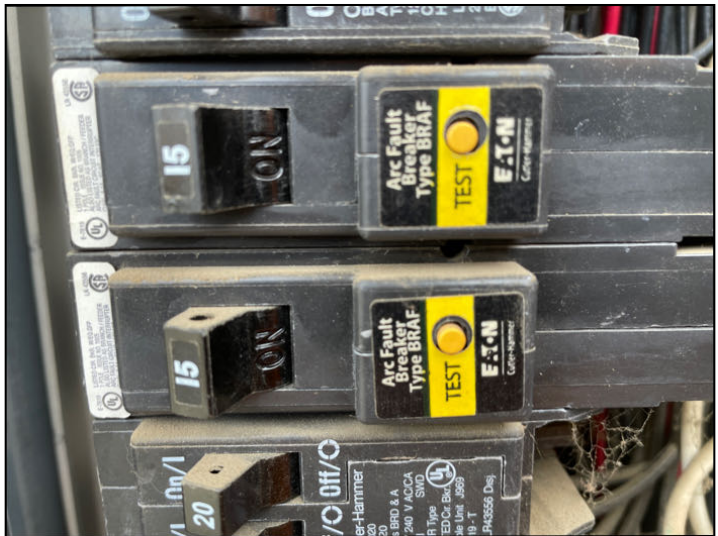
AFCI Breakers. Tested. Operated correctly.
