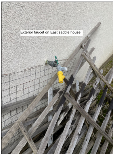
Recommend removal/relocation of extraneous materials to avoid damage to stucco, faucet, and prevent insects.
