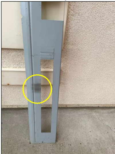
Heat marks from AFCI breakers
