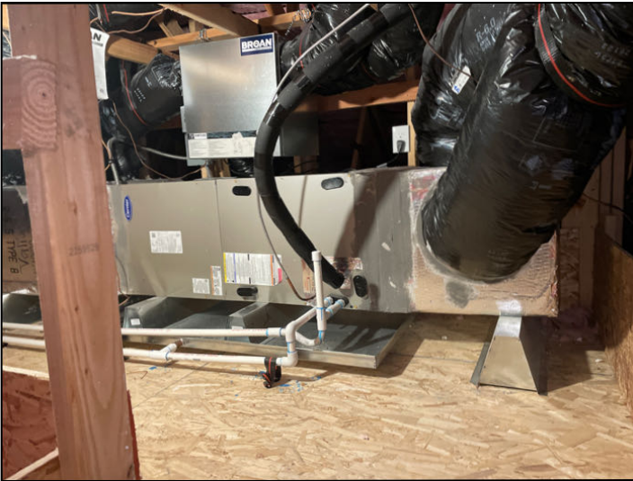
Attic heater. Functioned as designed when operated.
