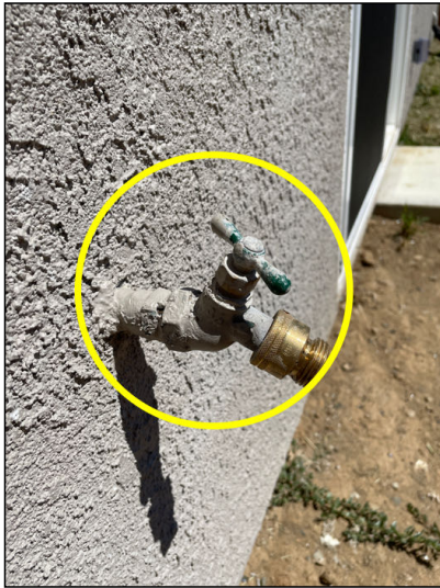
Exterior faucet at the rear of the structure was heavily painted over. This can cause damage to the seals in the fixture and create early failure. Recommend review by builder and repair/replace as necessary.
