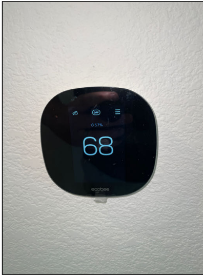
Digital, programmable thermostat located in hallway near the living room.
