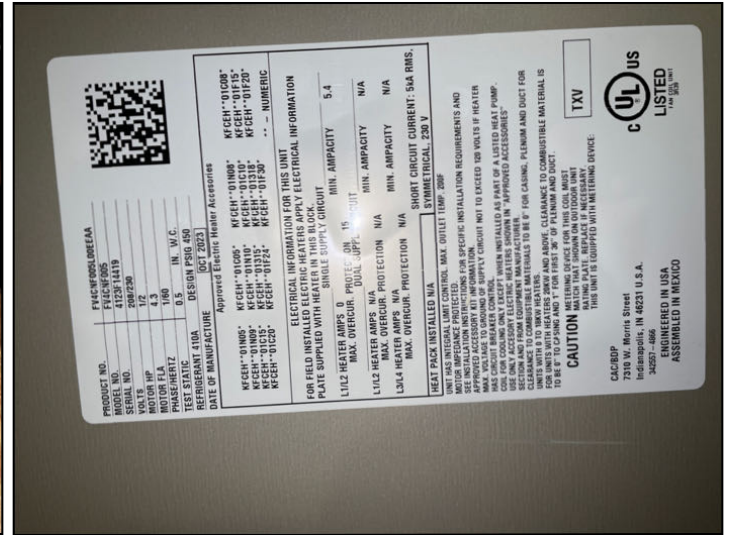
Carrier HVAC system in attic.
