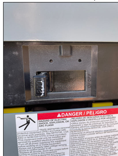
200 amp main breaker. Underground Service Lateral.
