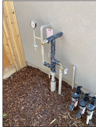
Northeast corner of house. Exterior faucet and water main line entry to the structure.
