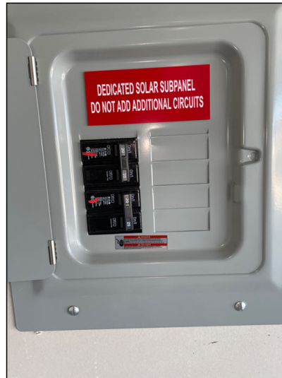
PV sub panel located in the garage.
