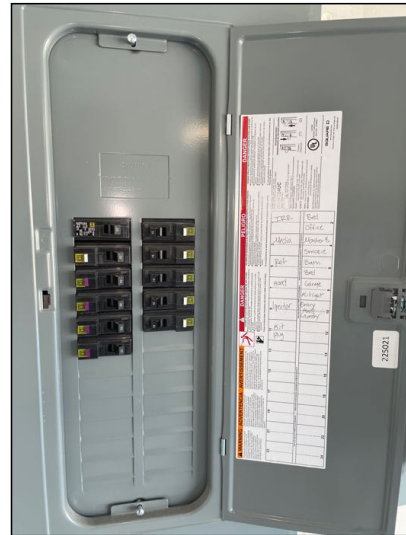
Sub panel located in garage
