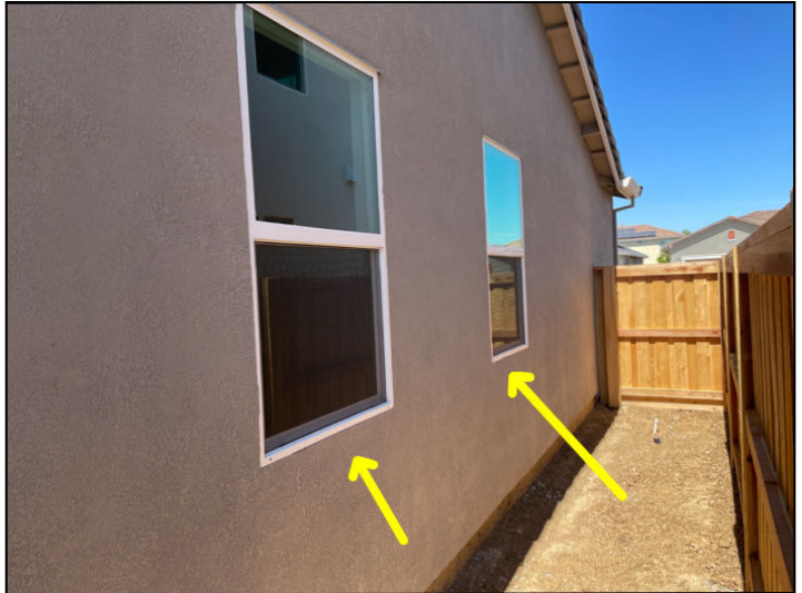
Windows on the east side of the home are not fully caulked and sealed at the bottom. Suggest further review by the builder to ensure all the windows on the exterior are fully caulked and sealed.
