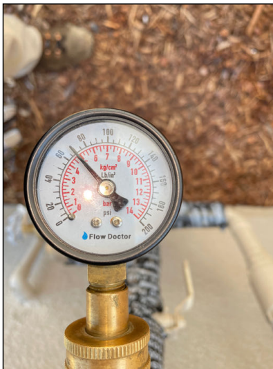
Water pressure at exterior faucet at the northeast corner of the structure showed 70 psi.
