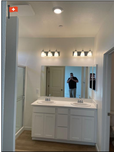
MBR Bathroom. See additional photo and caption regarding incorrect placement of receptacle near the shower.
