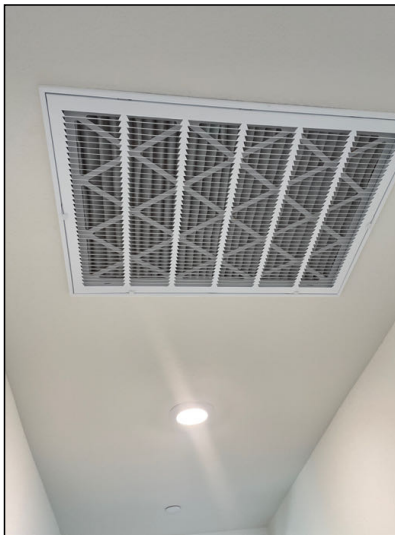
Hallway. Return air filter.
