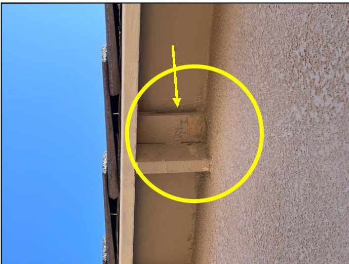
Eave boards unpainted and large gap. This provides accessibility for rodents, insects, and other nesting fauna. Blowing rain can collect in the open gap and hasten deterioration of board and roof deck, creating larger problems in the future.
